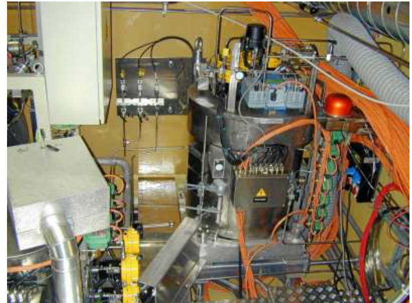
decay tank box in TKE
